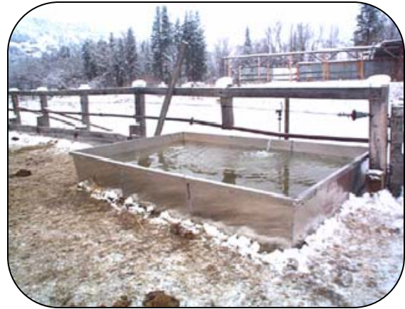
One of the troughs installed as part of a project to restrict cattle access to the Kettle River.
